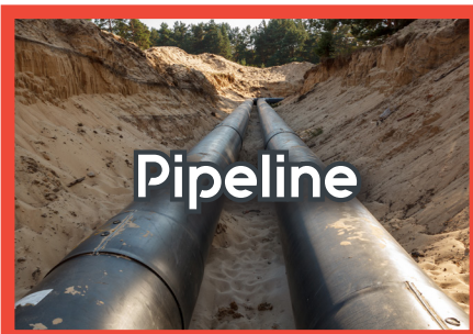
A pipeline carries oil or natural gas.
